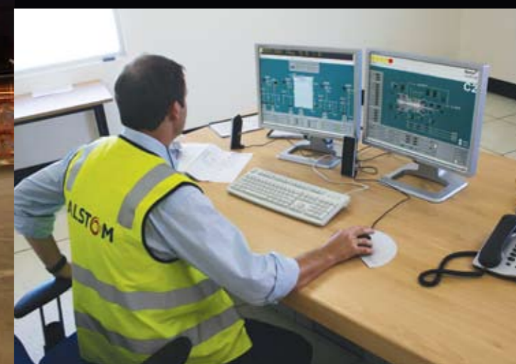
The power station can be started with the click of a computer mouse and remotely controlled from Delta Electricity's corporate office in Sydney, 120 km away.
